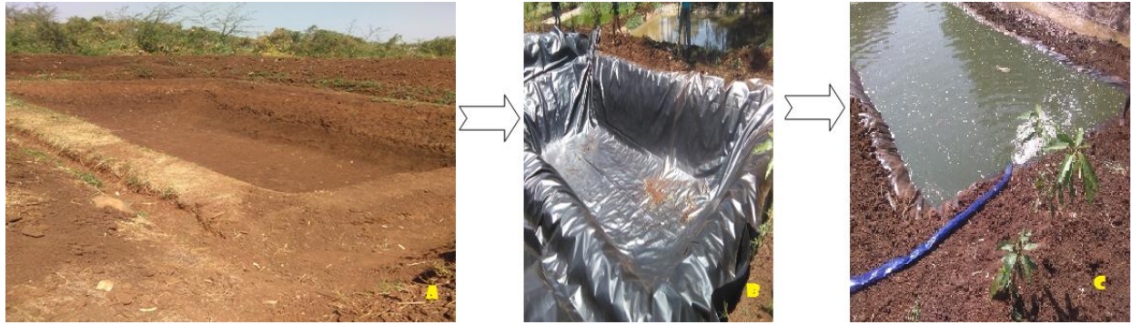
Figure 2. Photos show that the constructed (a), geomembrane lined (b) and ponds filled with water (c) during the experimental days.
